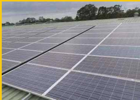
Werombi NSW 100 kW system Date of install – January 2015
