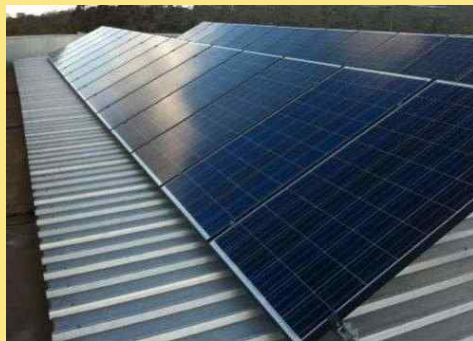
Highfields QLD 7kW system Date of install – September 2014
